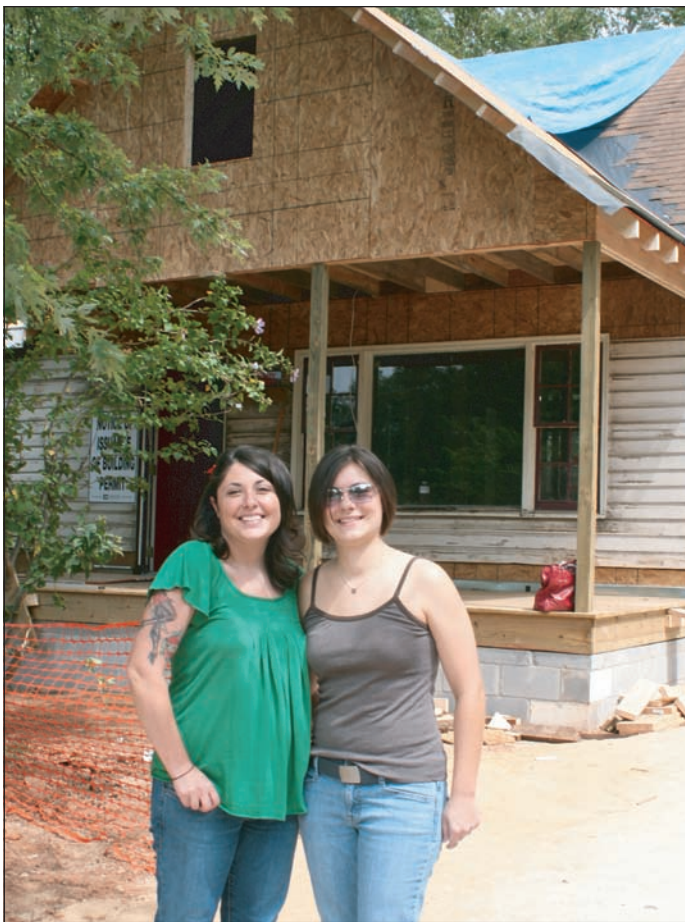
Rebecca Taub, left, and her partner Brenda Plympton stand in front of their Reynoldstown home undergoing renovation.
